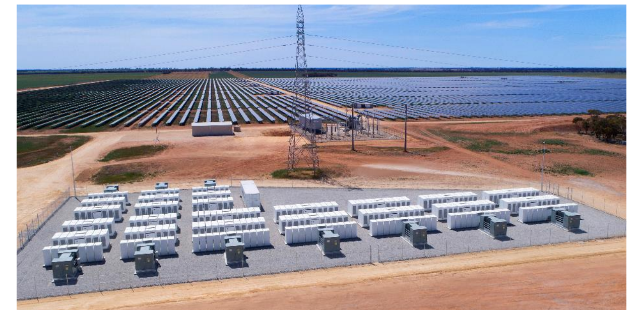
Commercial Solution: Solar and Storage
